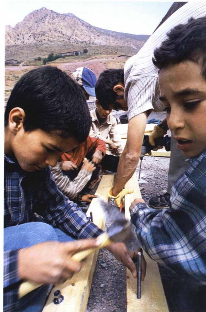
Students help construct rafters for the roof of their new school. All the building materials for the school, a collaborative effort by local residents and American climbers, were brought to the village on donkeyback.
